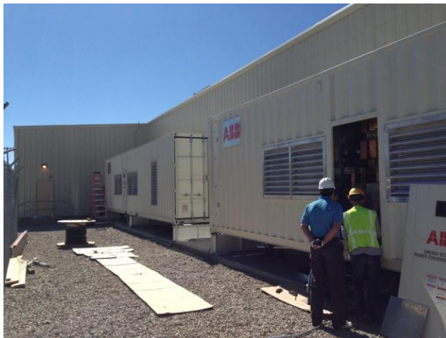
8 MW / 32 MWhr Tehachapi Storage Project
